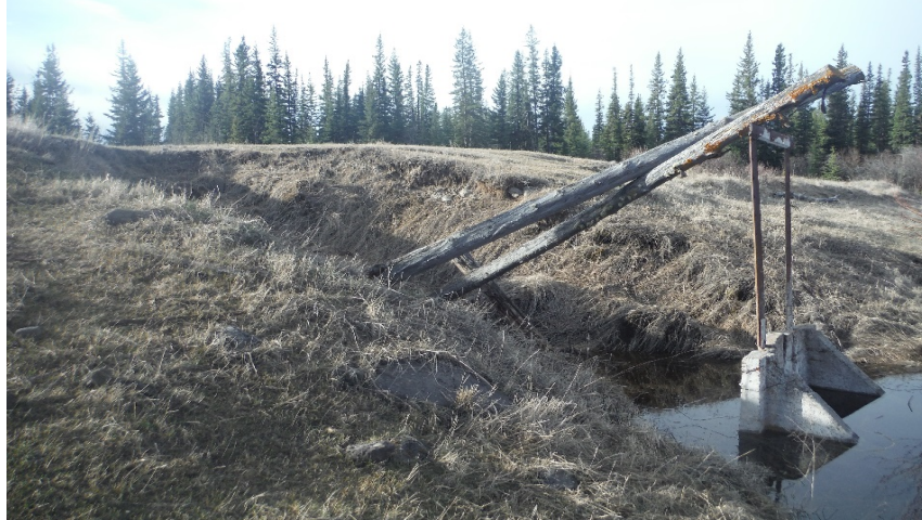
Figure 5: Failure at the outlet structure on the decommissioned Sword Creek Reservoir #2 dam.
